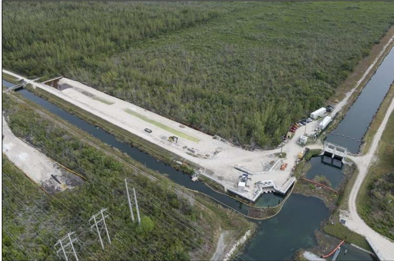
S-703 Pump Station and spreader system, December 2023
