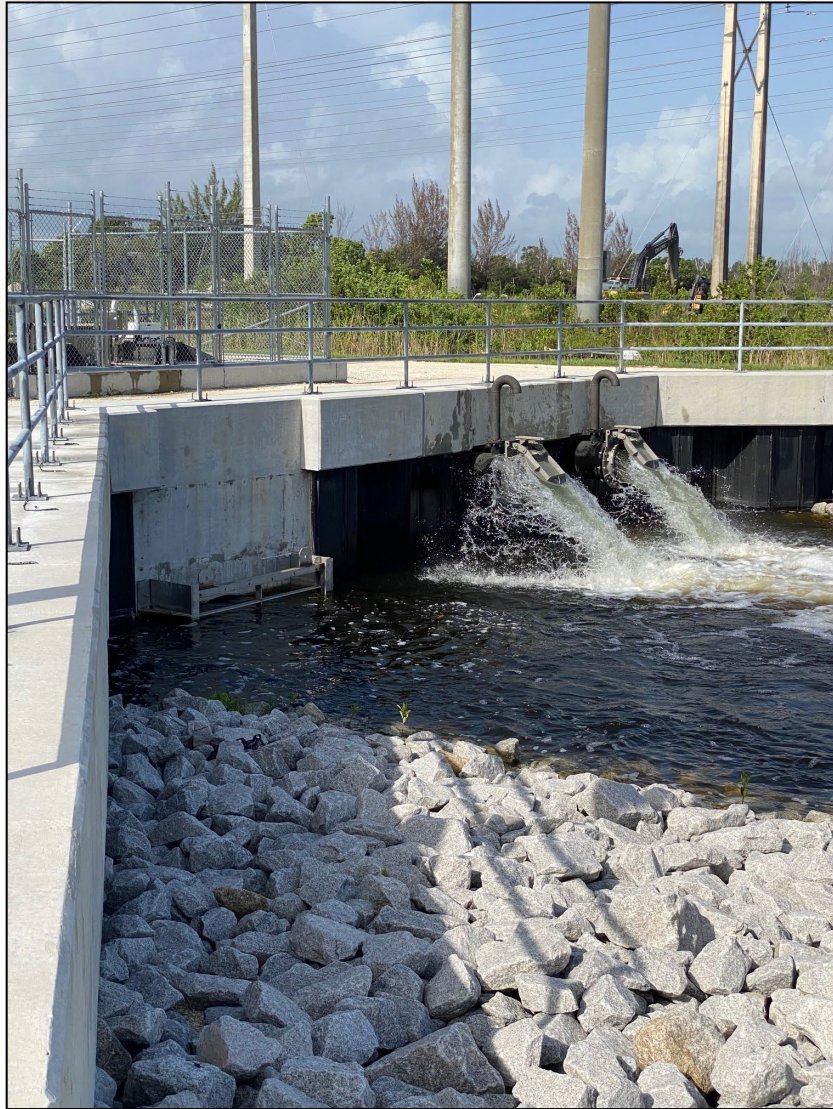
S-709 Pump Station, fully operational, Aug 2023
