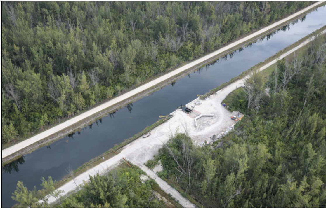
S-711 Pump Station, December 2023
