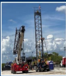
Mechanical Integrity Test at L63N
