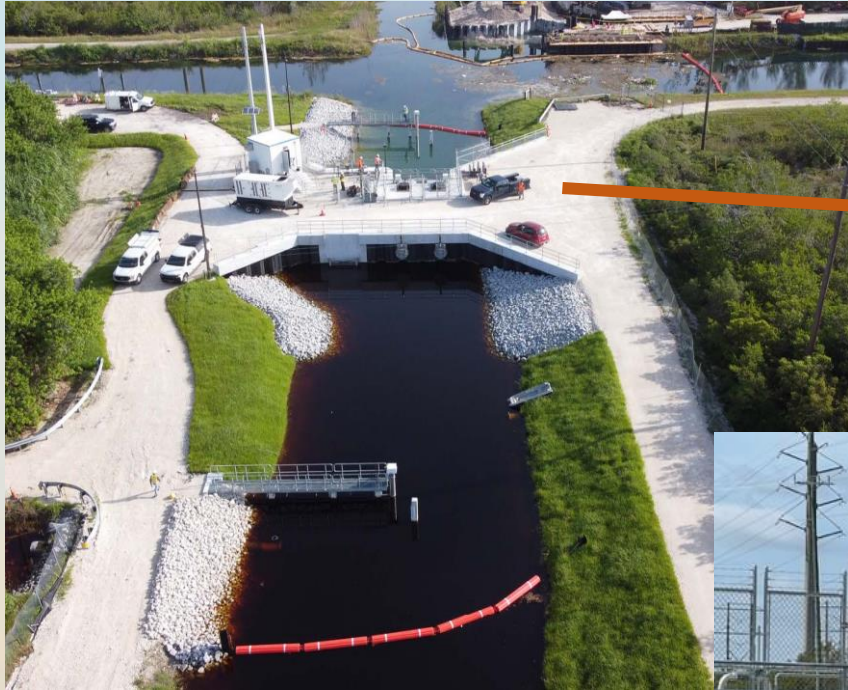
Pump Station S-705
