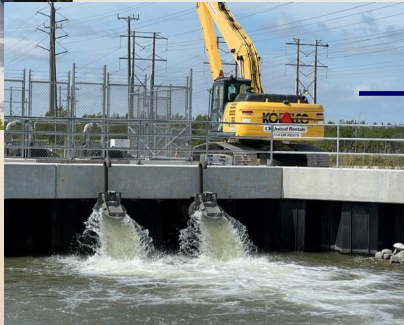
Pump Station S-709
