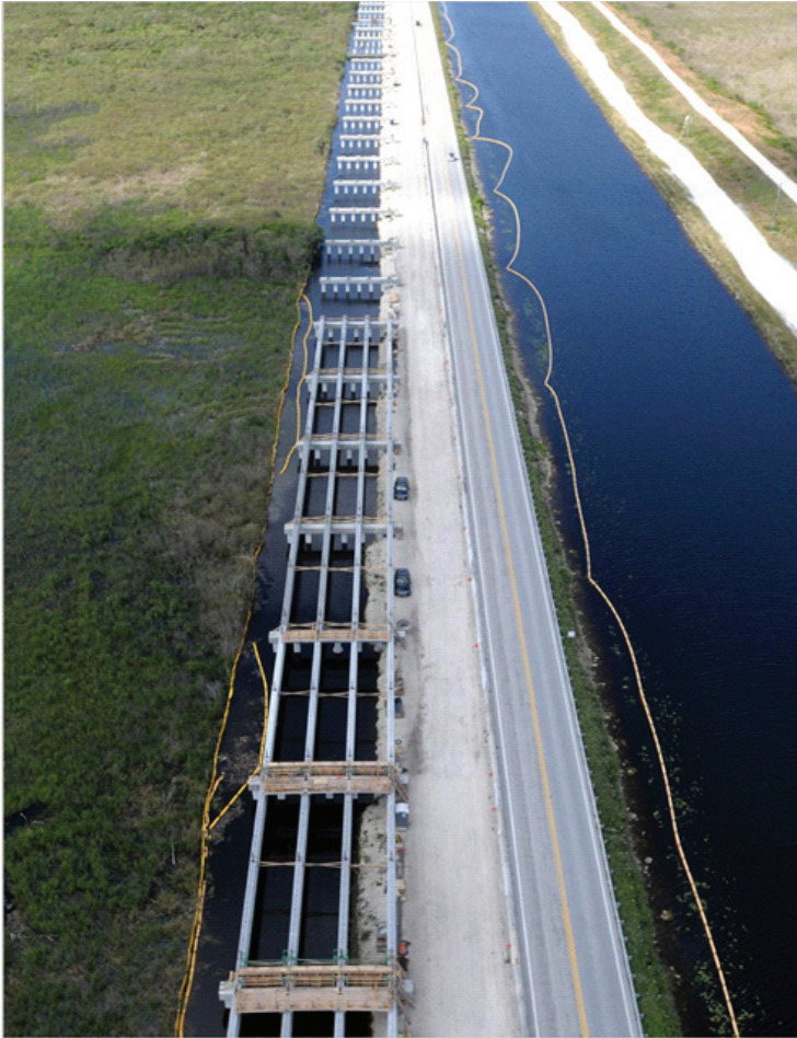
FIGURE 3-14 Construction of the Tamiami Trail 1-mile bridge, December 2011. From left to right, the image shows the north edge of Everglades National Park, the new bridge under construction, the Tamiami Trail (U.S. Highway 41), the L-29 Canal, its levee, and the surface of WCA-3B.
