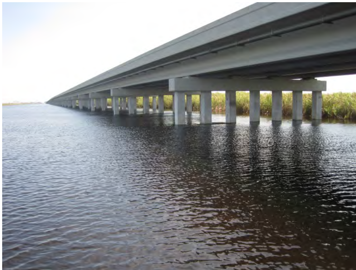
FIGURE 4-22 The newly constructed 1-Mile Tamiami Trail bridge, showing conveyance area beneath the newly elevated highway.
