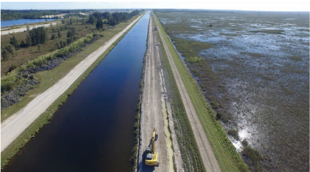
FIGURE 3-27 Southward-looking view of seepage barrier trench, excavated along the western side of L-31N.
