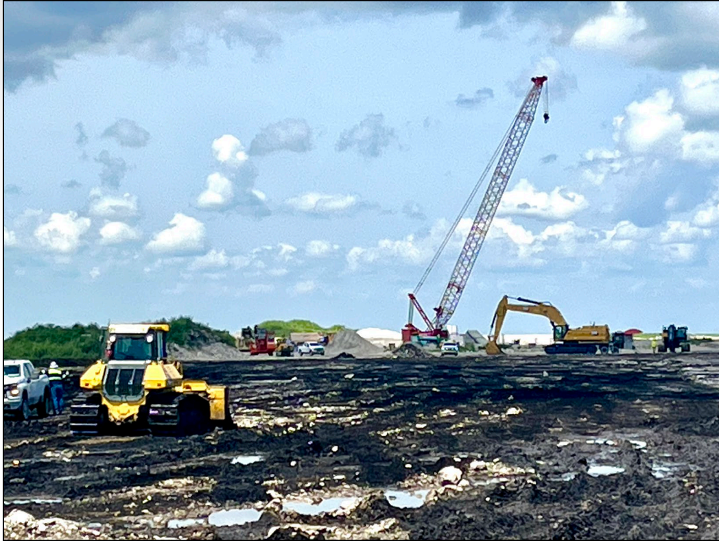
Everglades Agricultural Area (EAA) Reservoir, Construction of Inflow-Outflow and Seepage Canals Underway, May 2023
