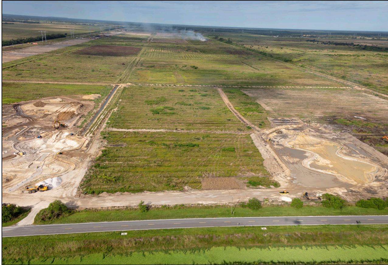
C-23/C-24 Stormwater Treatment Area, view west across Cell 5 (excavation underway for outlet structures S-439B and S-439A), October 2023
