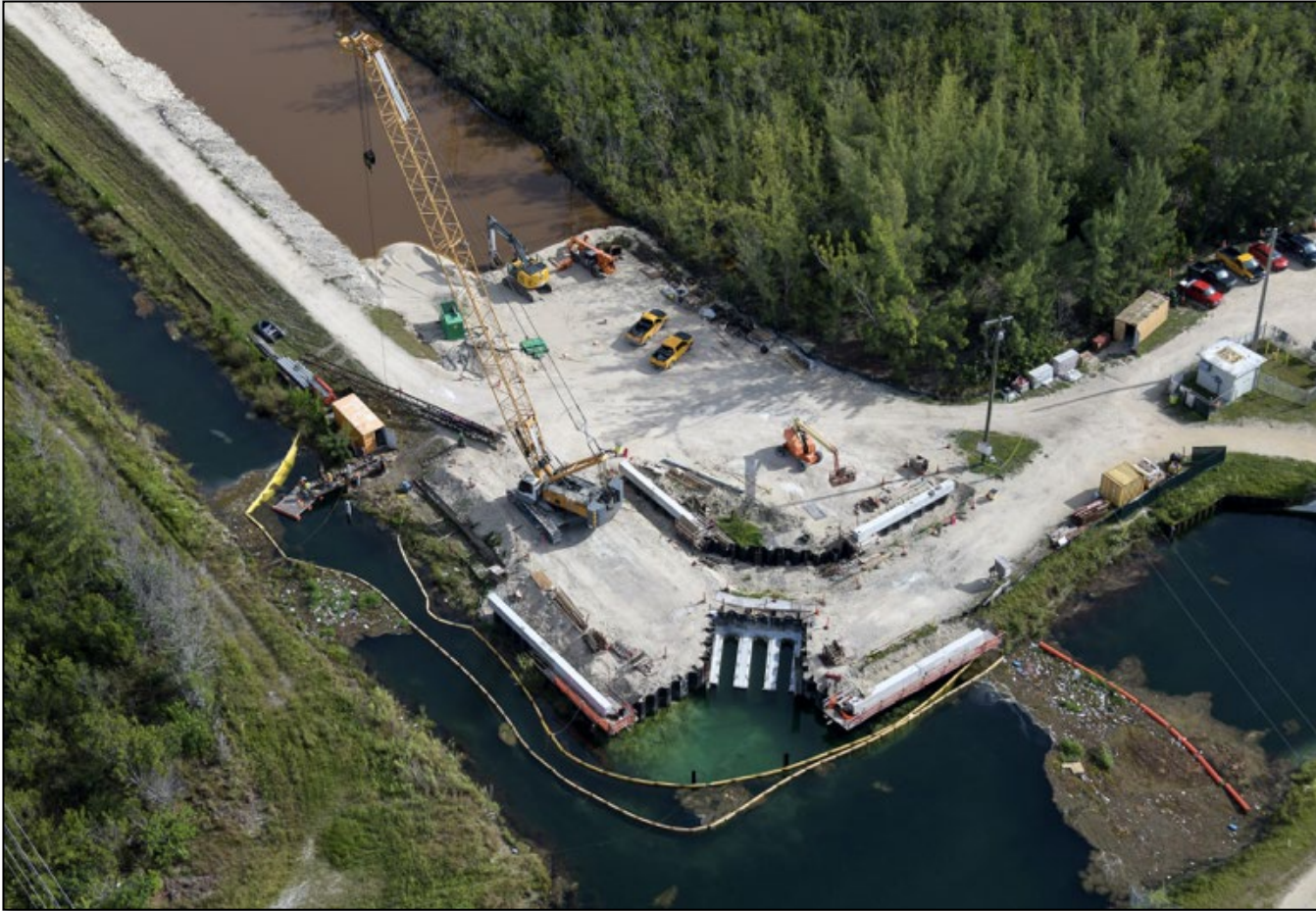
S-703 Pump Station, September 2023
